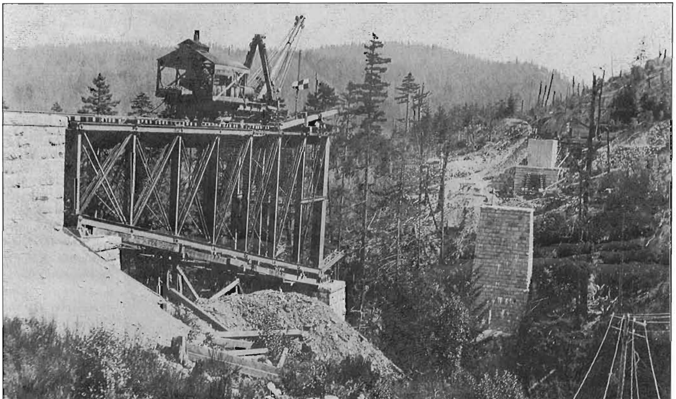
The Cisco Bridge has been dismantled and moved to the Esquimalt and Nanaimo Railway where it is being reassembled (and lengthened) over the Niagara canyon. CPR Archives # a26246
