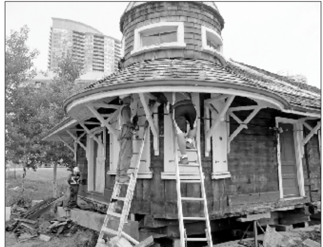
The Don Station, moved from Todmorden in December 2008, had the metal siding removed in preparation for a full restoration. Derek Boles
