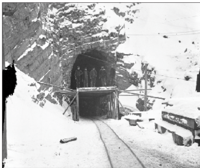
Workers on scaffolding at one of the spiral tunnel portals. Canadian Pacific Archives.
