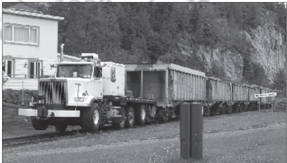
Contractor ballasting track on the Chemin de fer Charlevoix during the up-grade work in 2010. Denis Fortier.
