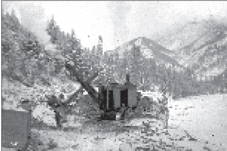
Great Northern's contractor steam shovel clearing a roadbed near Fernie, British Columbia. Okanagan Archive Trust Society, GNR 028, www.oldphotos.ca
