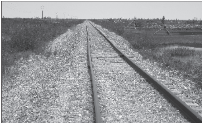
The HBR tracks across the tundra. The new electrical transmission line runs on the west side of the track, and the old transmission line on tripods to speed installation prevent falling over remain on the east side of the tracks. Peter Kevan.
