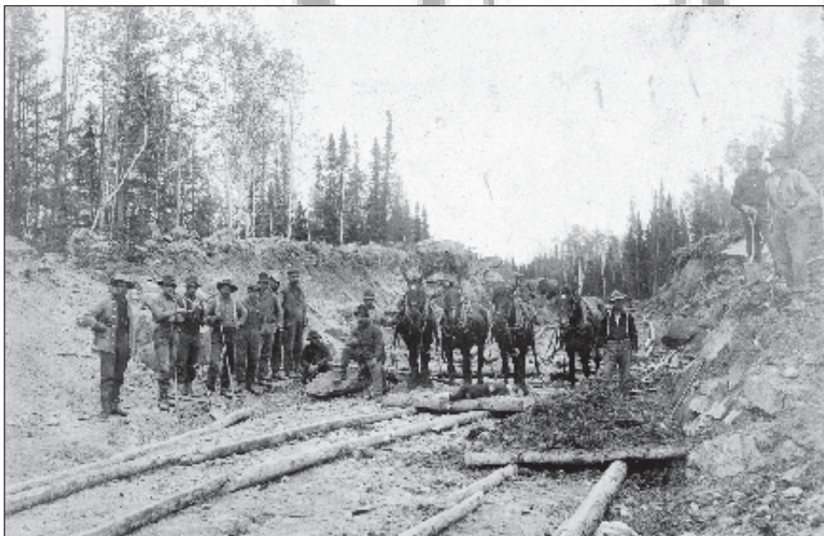
Grading the right-of-way in Northern Ontario circa 1908, it appears that the pole rails were used as skids for the wood platforms carrying material which were drawn by horses. Library and Archives Canada C-054478
