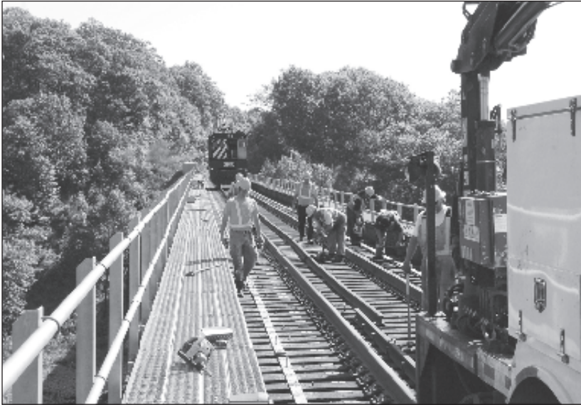
Crews are re-installing the guard rails after ties were replaced on the bridge in September 2009. John Soehner
