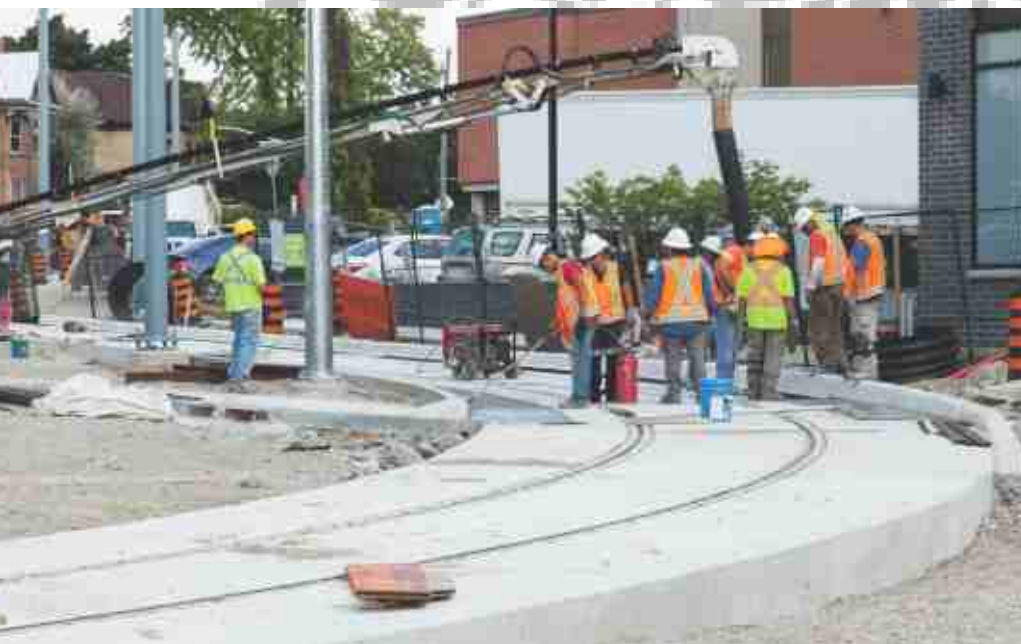
Three relatively recent shots of LRT construction progress. ION - Region of Waterloo Rapid Transit and John D. Thompson
