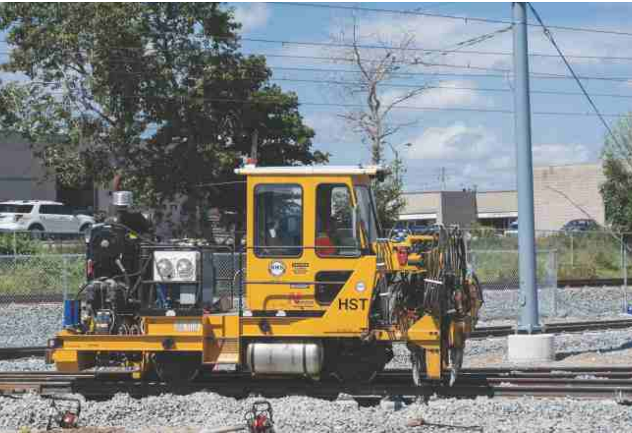
Tamper at work near the shop complex. ION - Region of Waterloo Rapid Transit
