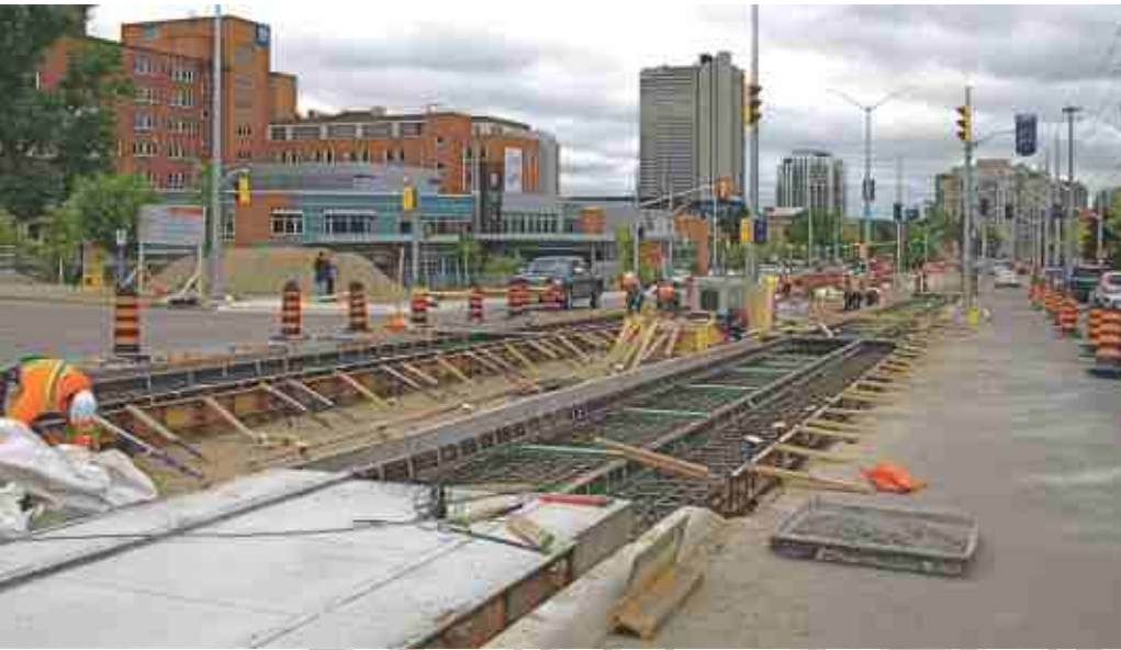
This view looks north on King Street just south of the important Grand River Hospital Station. Workers are preparing the reinforcing mesh prior to cement pouring. John D. Thompson
