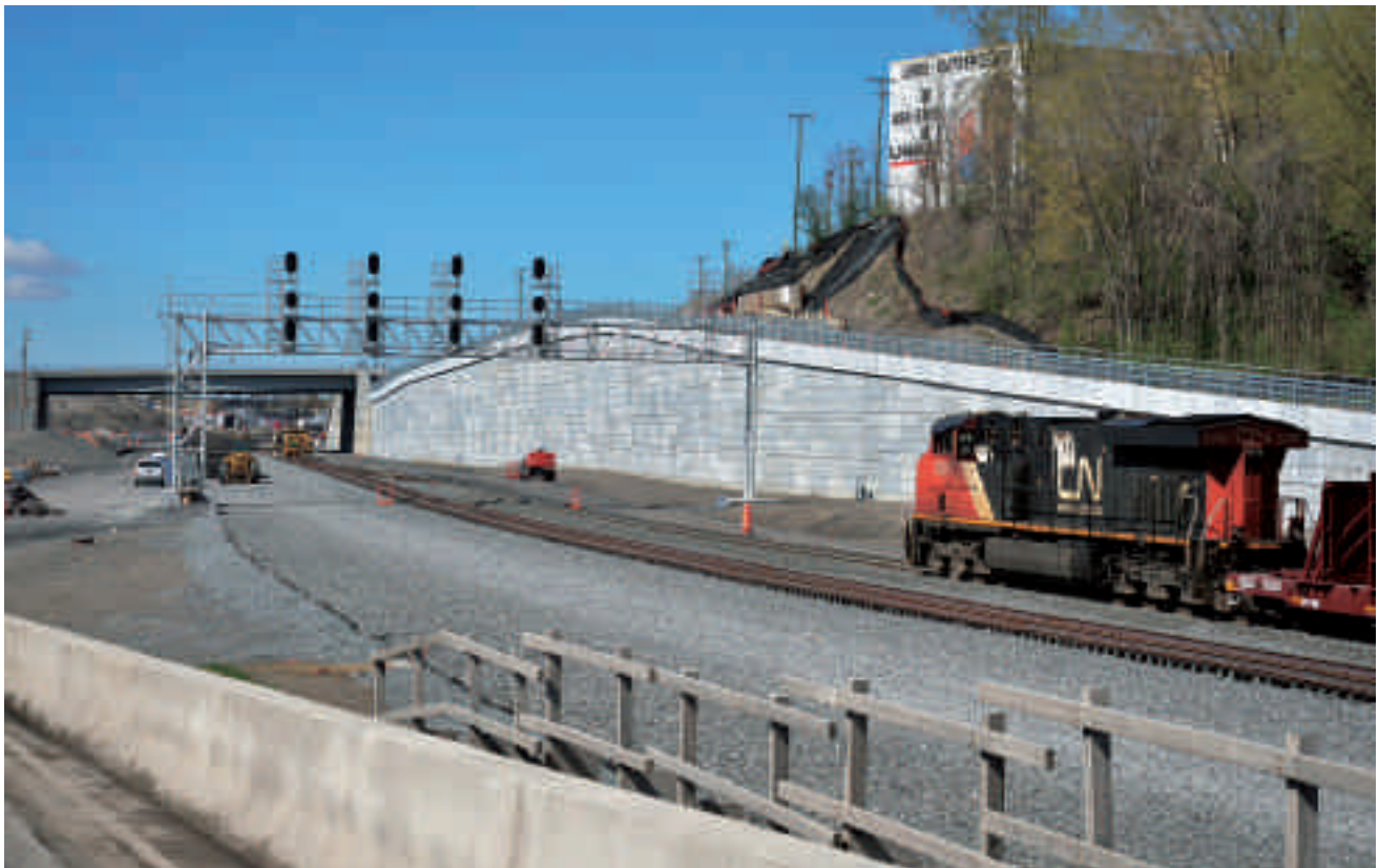
View looking west; the retaining wall is now complete and one track is laid May 12, 2017. Ken Goslett
