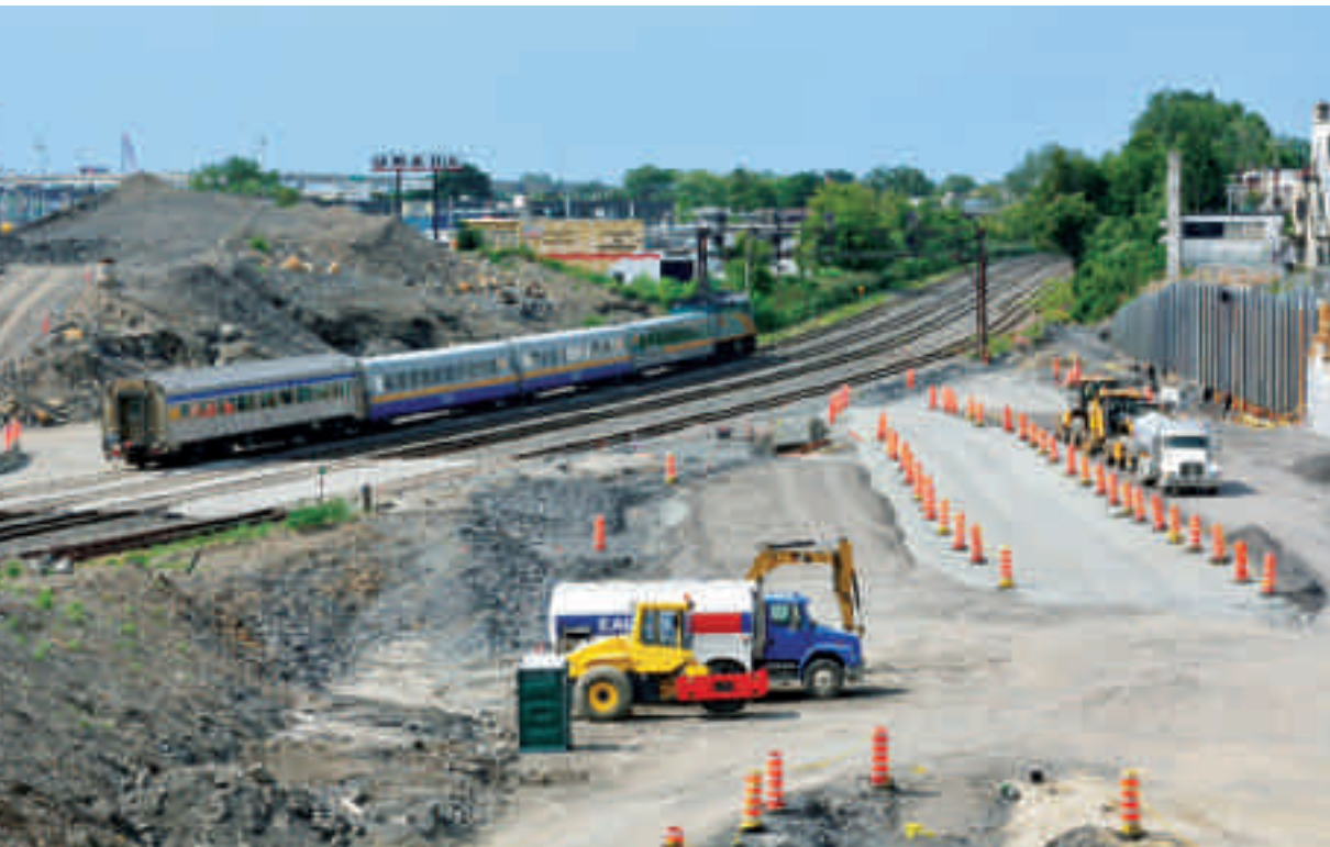
View from over the new right of way looking west at the west end of Turcot on August 21, 2016. Ken Goslett
