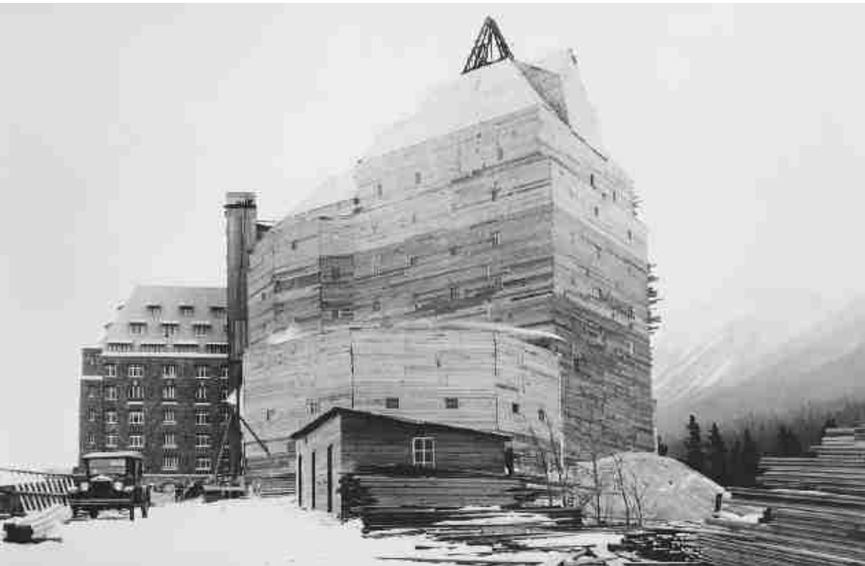
Enlarging the Banff Springs Hotel in 1926. CRHA/Exporail Archives, Fonds Canadian Pacific A2027
