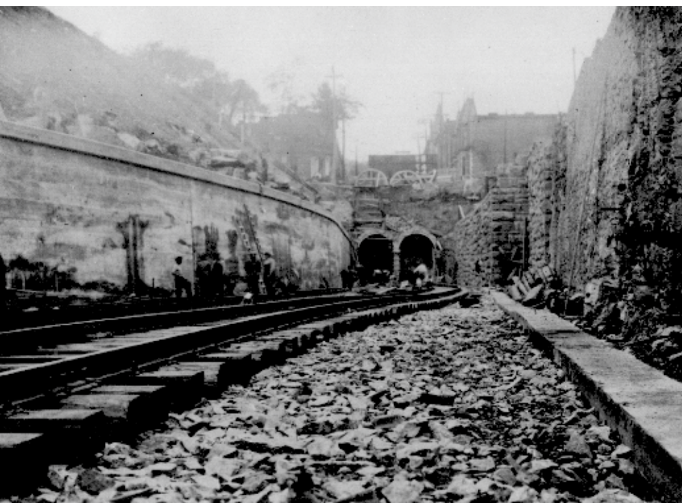
Initial tracks leading into the Mount Royal Tunnel's south portal in 1918, the tracks are yet to be ballasted and the overhead catenary has not yet been installed. Canada Science & Technology Museum, Fonds CNX-48579
