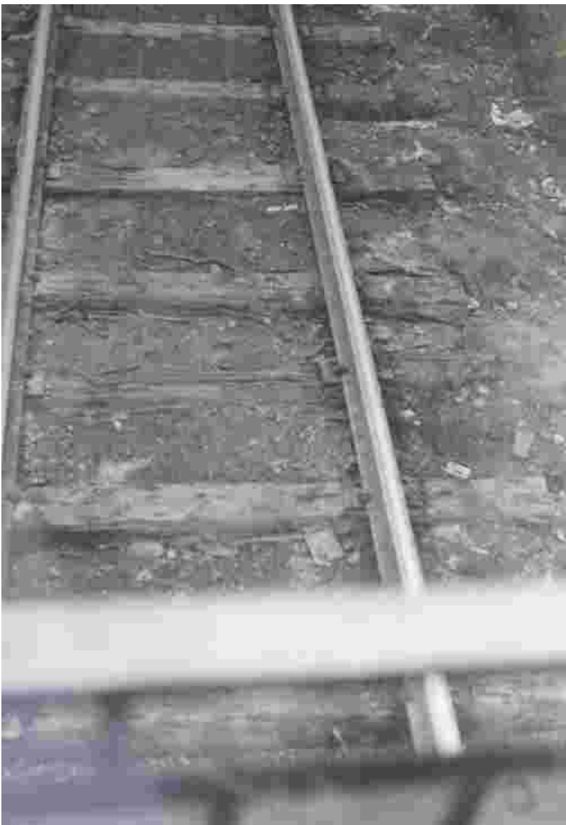
Photo 151: Decayed ties at Grand Falls.
