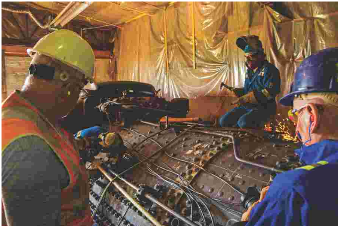
Three employees hard at work on top of 6060's boiler. Note the chalk grid on the boiler surface to help with the metallurgical testing. Jason Sailer
