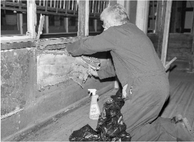
Terry Thompson removes horsehair insulation from walls of Regina streetcar 42 accompanied by plenty of dust. (Don Scafe)
