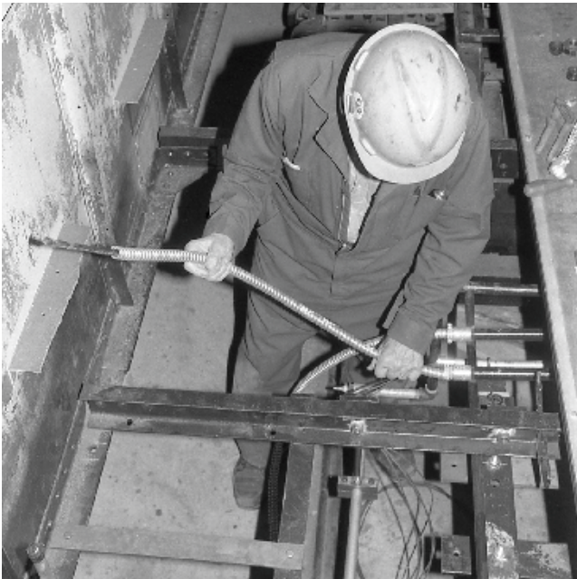
Arnold Rumbold prepares wire for a flexible conduit cover to Regina 42 line-breaker. (Don Scafe)
