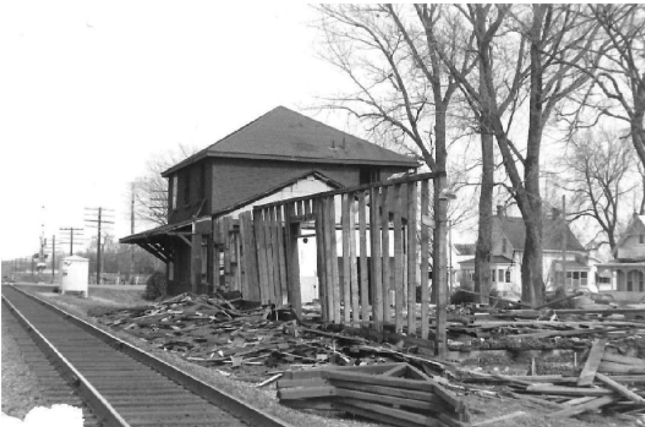
The demolition gang made short work of the Mountain station in the late 1970s. Railway Museum of Eastern Ontario
